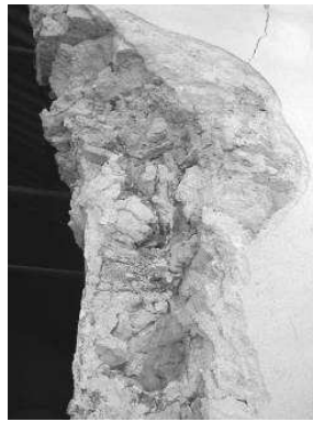
Figure 3 Only some spots were injected in the case of this wall with a very low percentage of voids.
