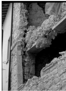
Figure 2 Effect of eccentric loading due to RC tie beam positioning.
